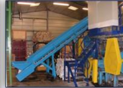
STOCK PREPARATION Vitry, France
